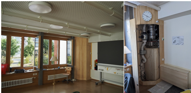
Ventilation in the classroom, air is sucked through the porous tubes at the ceiling, filtered and recirculated by the channel below the blackboard, right: filter and blower.
